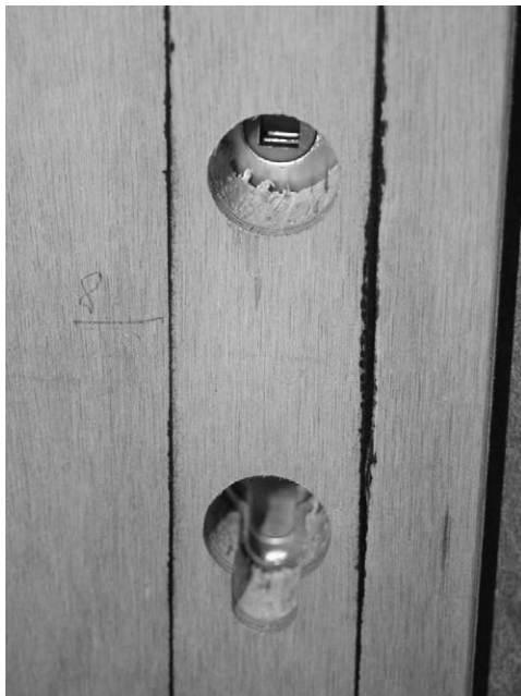
Fig. 7. Cylindrical hole accommodating the pin in door leaf facing after removing doorplate.
